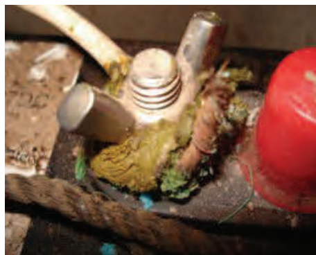
Figure 10. Corrosion on battery
